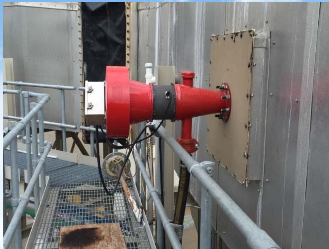
Tri-Mer Injector installed in UCF system duct
