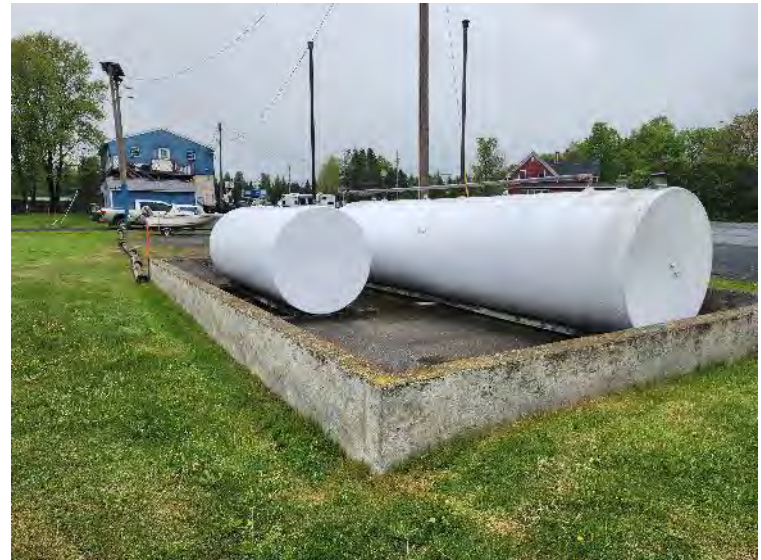
Gasoline ASTs, concrete dike in south yard
