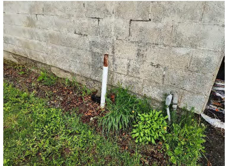
Two buried 1.5-inch steel pipes, possible UST?
