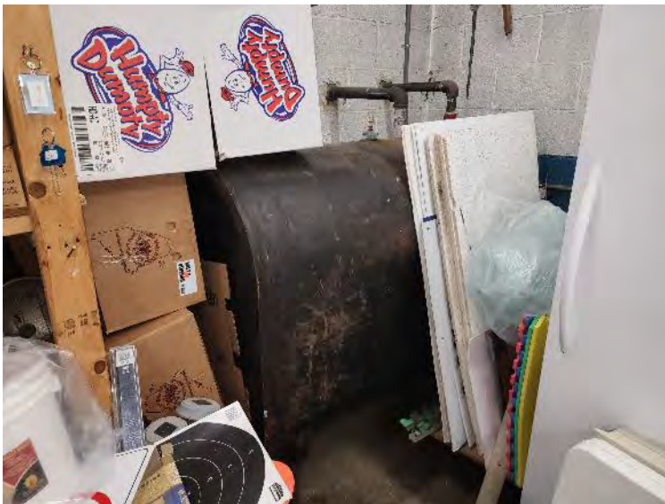
275-gallon fuel oil tank in southwest corner of garage
