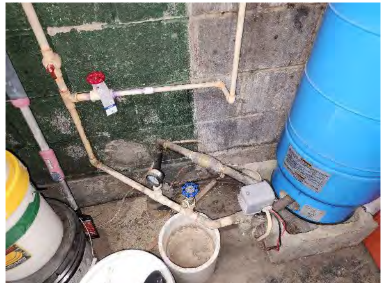
Expansion tank, water supply point of entry
