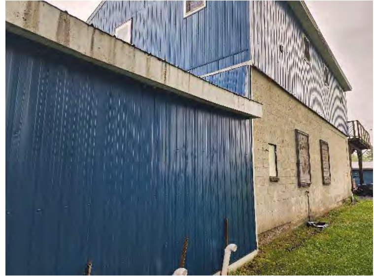
PVC vent pipes, west side of commercial building looking southeast
