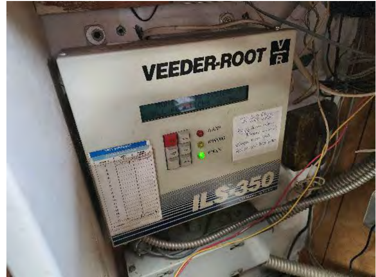
Transition sump leak detection monitoring console
