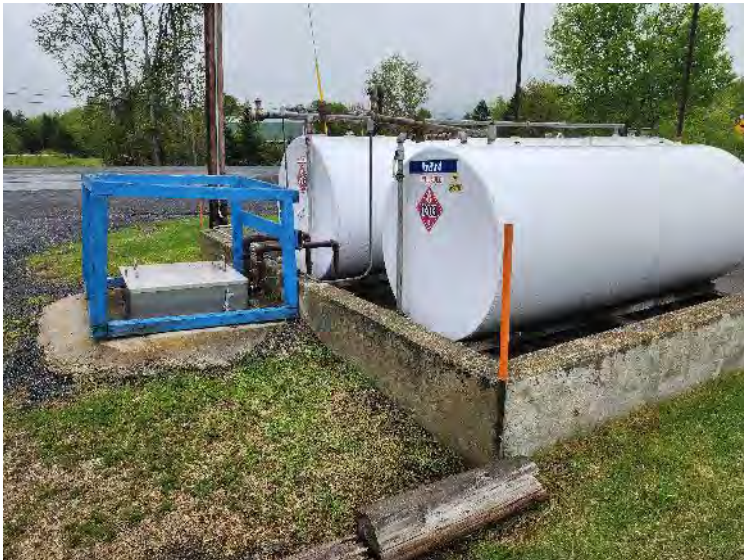
Gasoline ASTs, transition sump south in south yard
