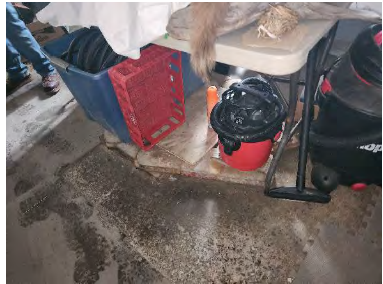
In-ground hydraulic lift, garage bay
