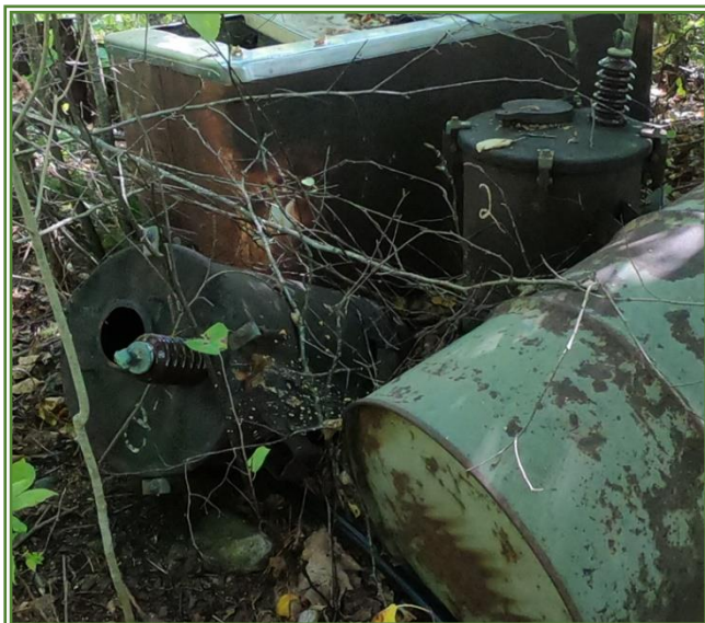
Two Transformers each wipe sampled
