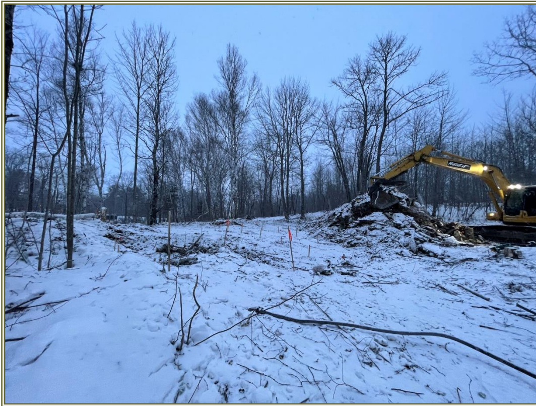
PCB-impacted soil pile
