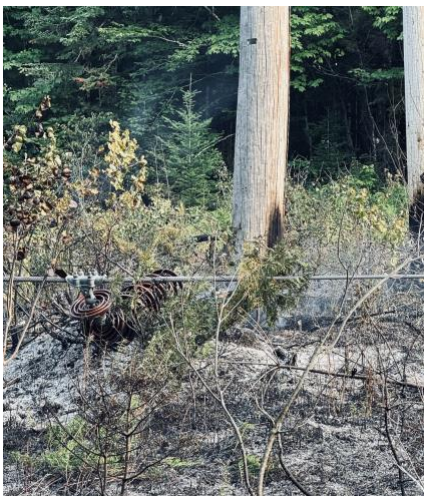
Broken, scorched insulator string on the ground amid burned understory vegetation.
